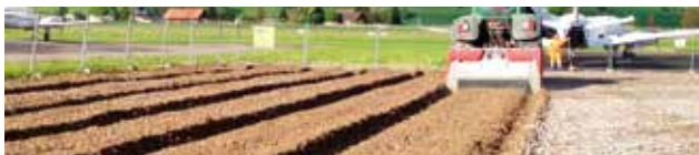
Vegetation base layer through soil improvement: Milling of gravel into the existing topsoil
